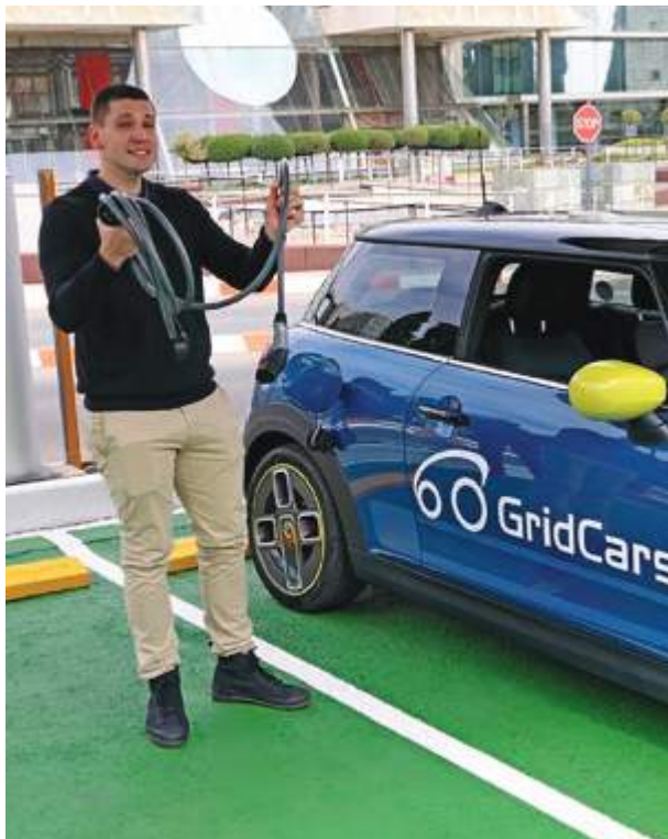
Electric vehicle charging station at the Vodacom Midrand campus.
